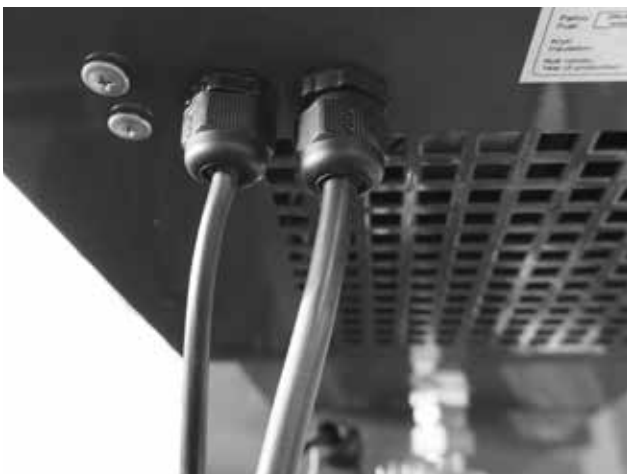
Fig. 11 - connection of electric valve and comperssor for pellet burner pneumatic ash cleaning system
